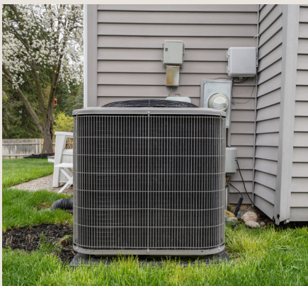
Central HVAC System
