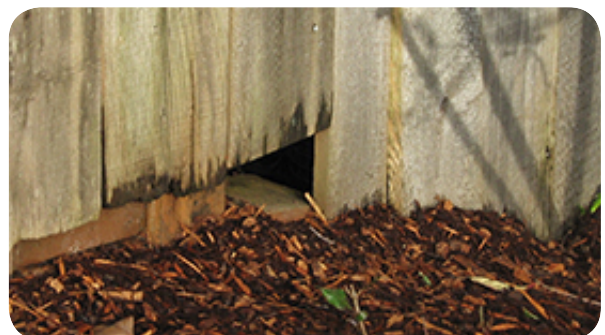
Gap under a fence
