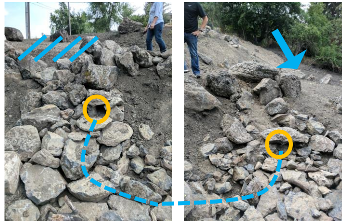
Figure 2. Sheet flow runoff is received from the road above and conveyed through a series of vegetated swales and pipes before ultimately discharging to a catch basin. An overflow pipe from a ravine is also connected to the system for additional capacity during high rain events.
