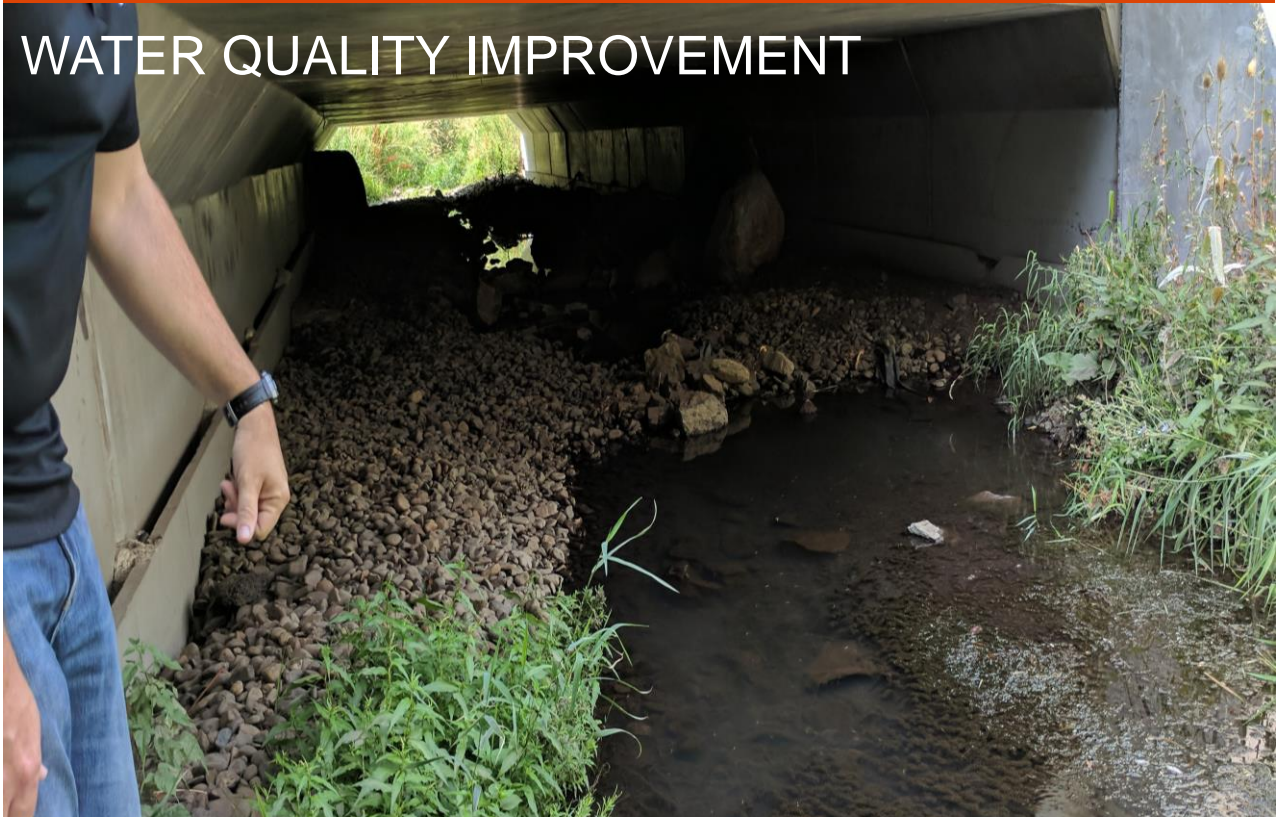
Pictured above Kyle Carpenter (Environmental/Regulatory Superintendent) showing where the LID swale outflows into Gekeler Slough.
