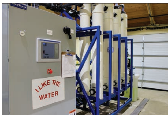
Photo: Emily Jane Davis, © Oregon State University Figure 9-15. Membrane filtration system in the Oceanside treatment plant.
